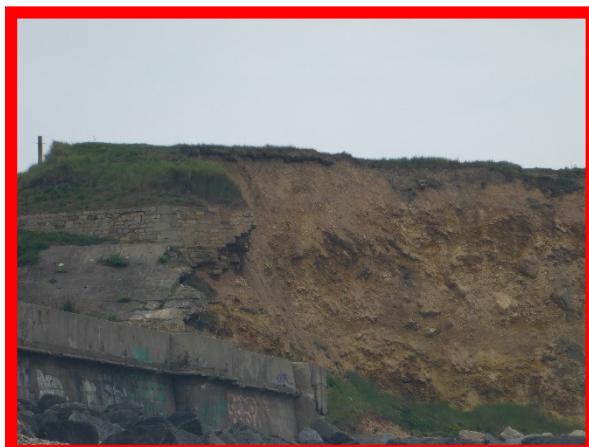
Masonry wall and concrete revetment at tie-in to cliffs breaking-up (/0103C04)
