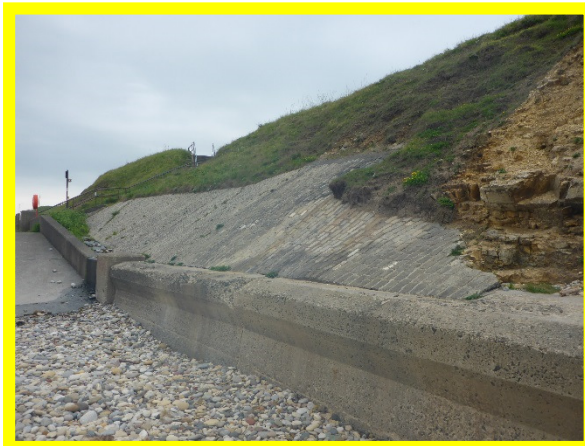
Minor outflanking of blockwork revetment (/0102C01)
