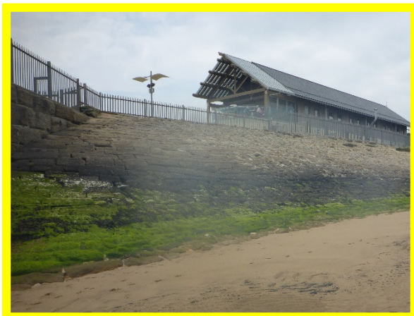
Open joints and vegetation growth on masonry revetment (/0104C05)
