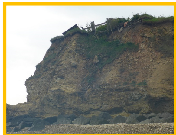
Erosion affecting fence line of properties to south of Dawdon Dene outfall (/0103C02)
