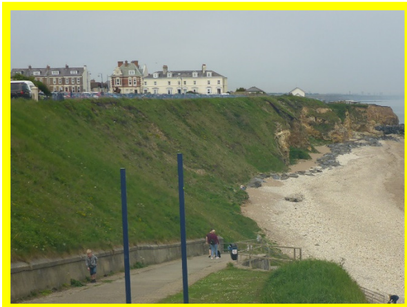
Local slumps in cliffs (/0103C06)
