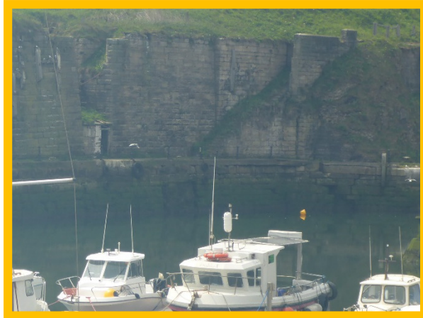
Gaps between blocks at Seaham North Dock (/0104C12)
