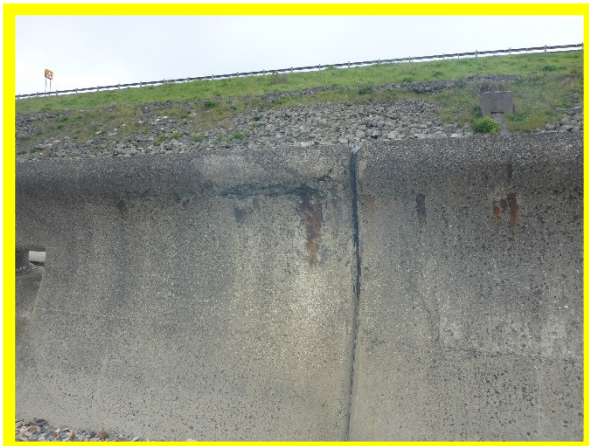
Spalling of bullnose on sea wall (/0102C01)
