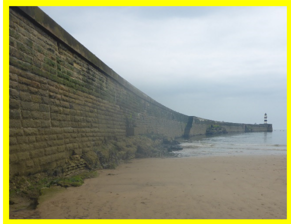
Seaham Harbour North Pier Inner Face (/0104C03)
