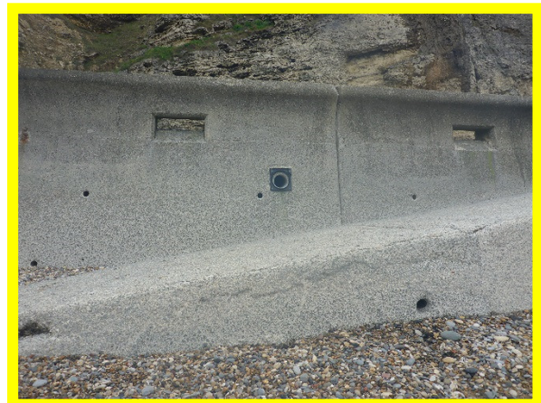
Missing flap valve at access ramp (/0102C01)
