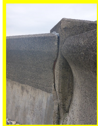
Sealant missing at joint between sea wall and access steps (/0102C01)
