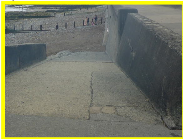
Cracks in deck of access ramp at southern end of promenade (/0102C01)
