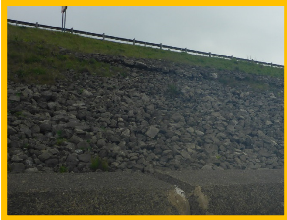
Remedial works needed to 'sunken' area of stone infill (/0102C01)
