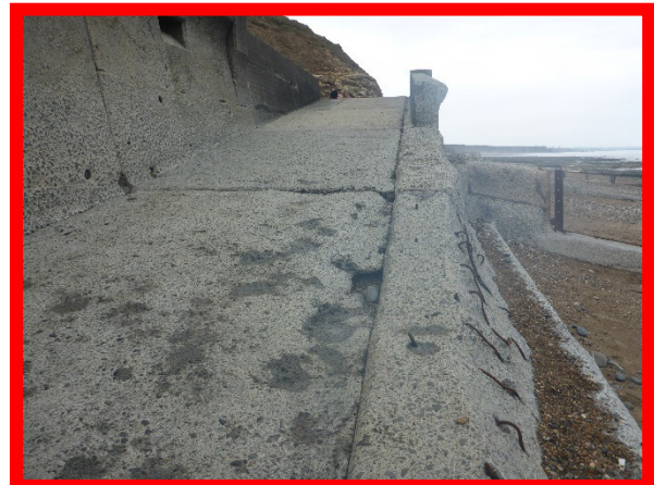
Hole in deck of ramp, exposed reinforcement (/0102C01)
