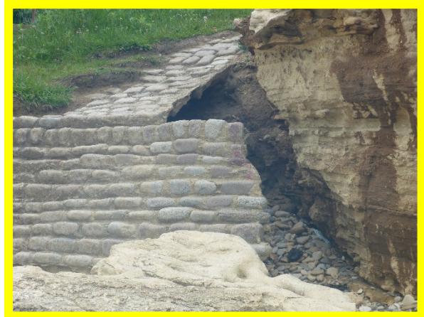
Outflanking of revetment (/0804C01)
