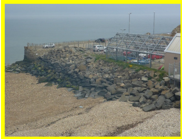
Low spot in revetment causing erosion to bank (/0103C07)
