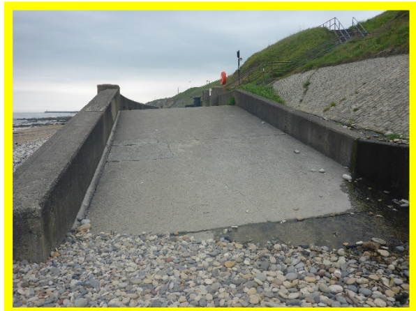
Cracks in deck of access ramp at northern end of promenade (/0102C01)
