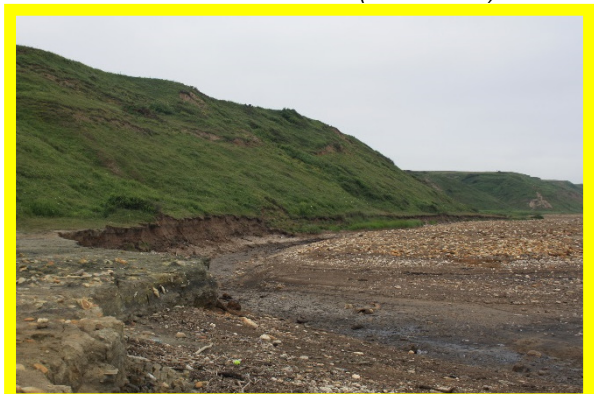
Undercutting at toe of coastal slope from mouth of Castle Eden Dene (/0201C01)
